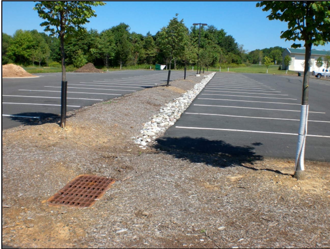
This parking area in Mountain Park has been designed with stone rows allowing better infiltration and recharge than standard curbing. Excess water is channeled to the catch basin located in the lower part of the photo.
